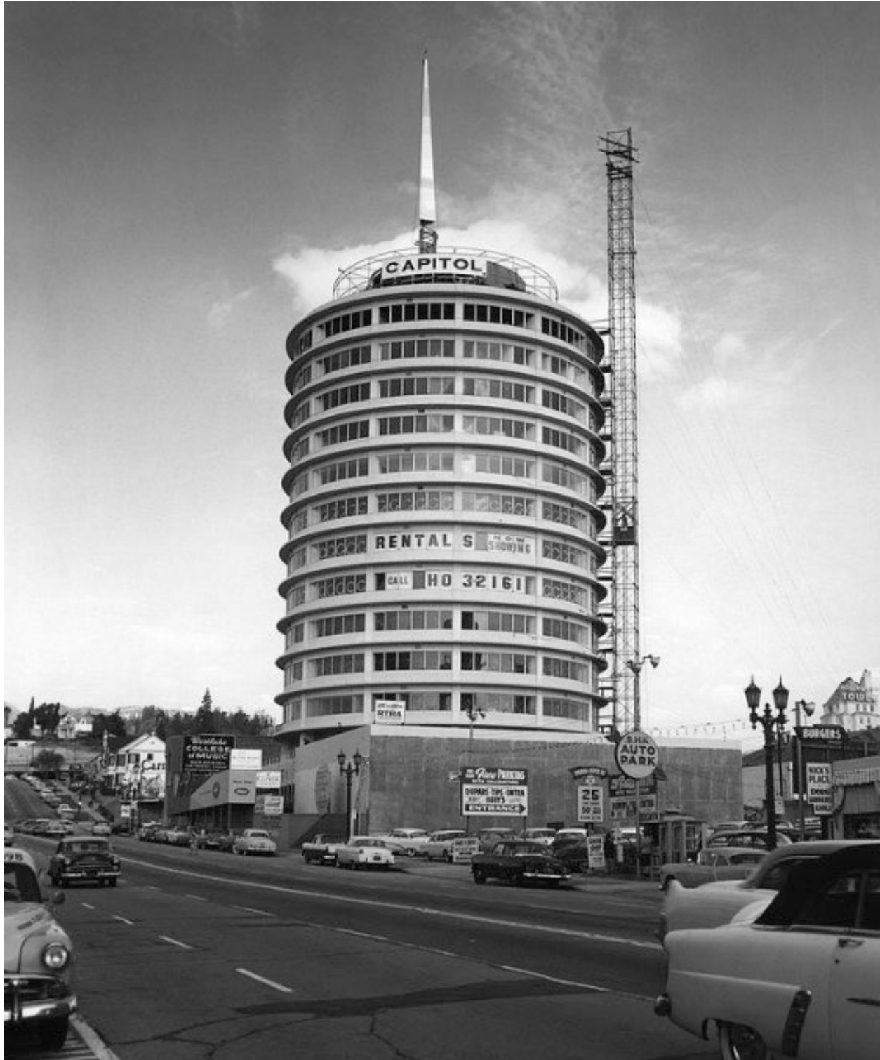
Figure 5: Capitol Tower near completion, view looking northeast from Vine Street, 1956. (Water and Power Associates)
