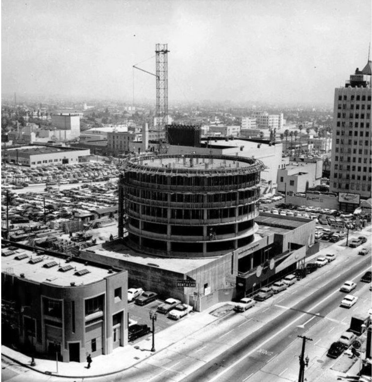
Figure 3: Capitol Tower under construction, view looking southwest from Yucca and Vine Streets, 1955. (Water and Power Associates)
