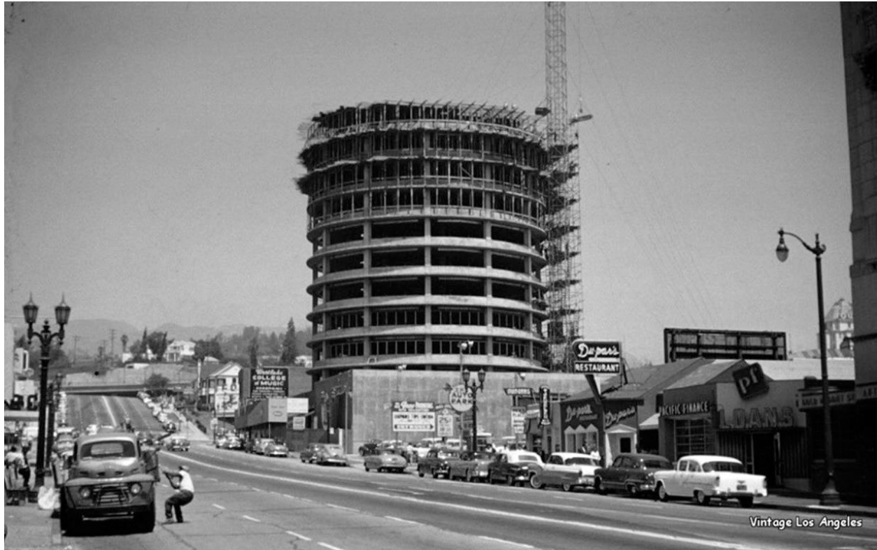
Figure 4: Capitol Tower under construction, view looking northeast from Vine Street, 1955. (Water and Power Associates)
